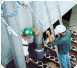
▲ Canada: water purification facility
