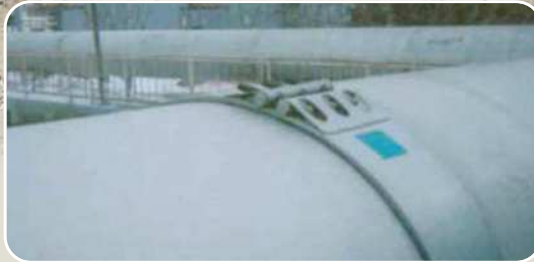
▲ 48" (1,200A) YNMF-RL Canadian power plant cooling line
