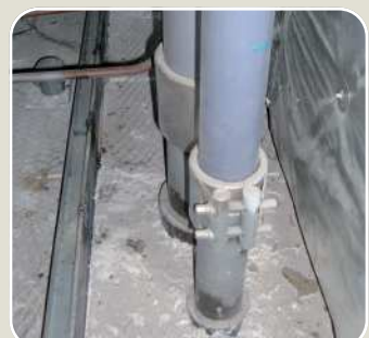
▲ PVC + Steel Pipe Connection
